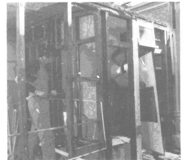
Workmen demolish a section of Corio prior to building a new office and store area.
